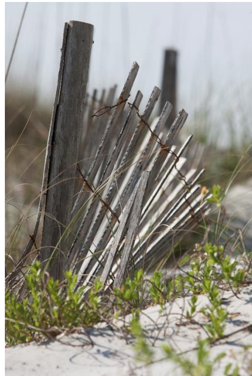
A wooden fence collapses among sand dunes in St. Augustine Beach, Florida. Credit: Tyler Jones, UF/IFAS
